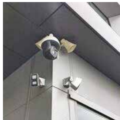
Elements of a Detector Activated CCTV system (camera, PIRs, loudspeakers)
